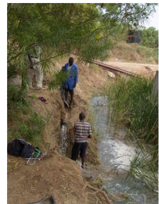
Biggest leakage since recording work of water leakage started.
