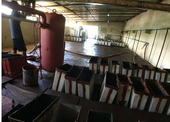
Ice plant in Shaplapur
