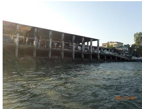
Cox's Bazar BFDC Ghat (Fish handling shed with collapsed north quay )
