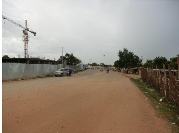
Photo 2-2-3 Current Situation of the Approach Road of Bridge No.7 (Completed until pavement)
