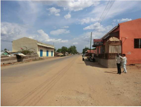
Photo 2-2-2 Current Situation of the Approach Road of Bridge No.4 (Completed until pavement)
