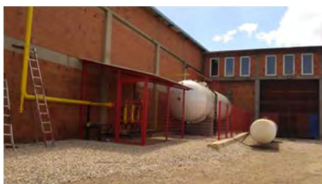
Photo 3-32 the supply facility of LPG
