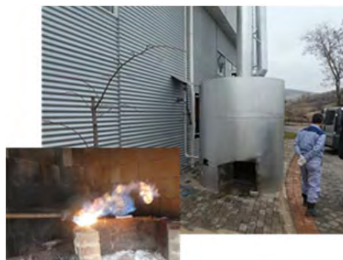
Photo 3-36 Combustion chamber for discharged gas
