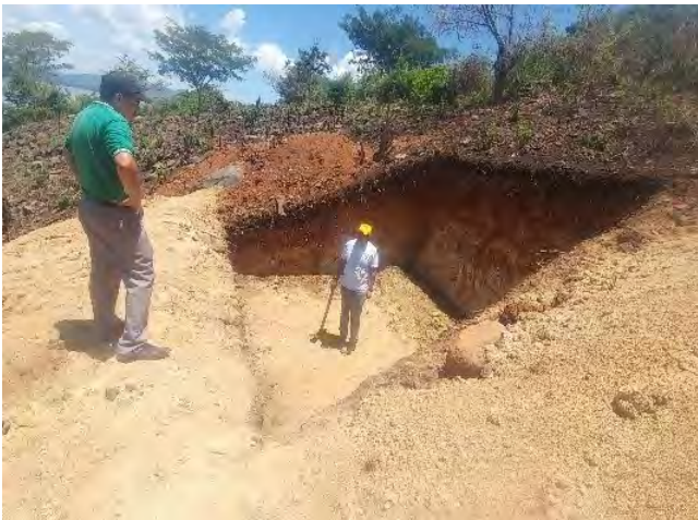
Photo 3: Construction of a reservoir in Canton La Estrechura Lagoon of Olomega. Here the layer is almost at a complete stage.
