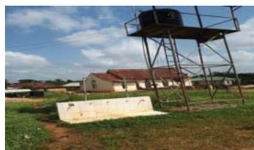
Plate 5.6 Borehole facility in Ekundayo
