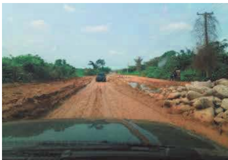
Plate 5.15: Devastating state of the major road
