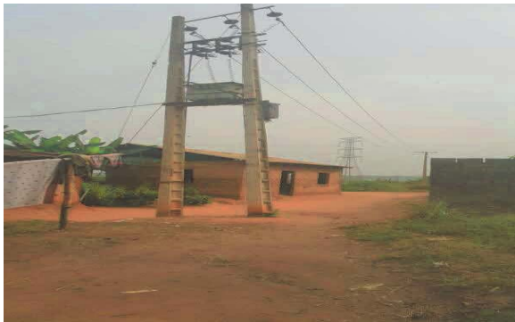
Plate 5.11: Electricity line and Transformer at Soderu Community
