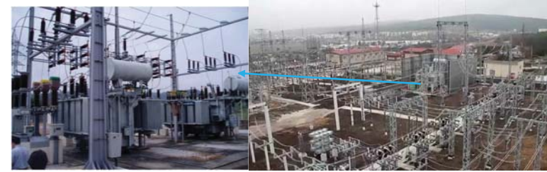
Figure 2.10 A Typical AIS Substation (with transformers zoomed in)
