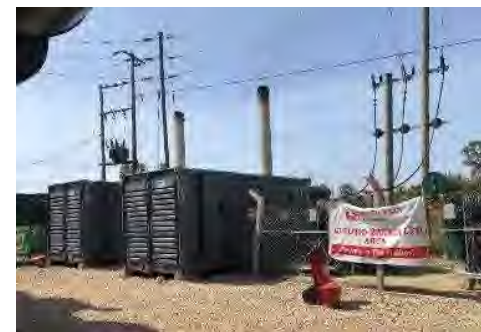
12 Diesel Generators, 8.2MW
