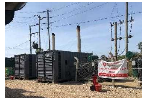
12 Diesel Generators, 8.2MW
