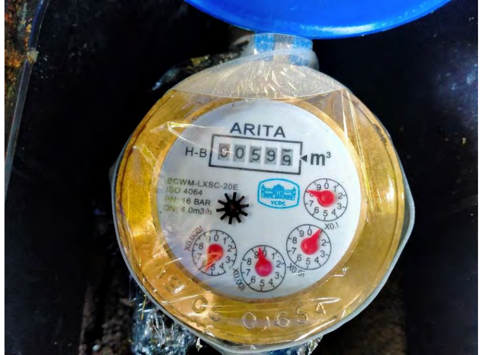
Water meter protection by plastic cover
