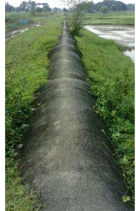
Phugyi Transmission pipe(Concrete)
