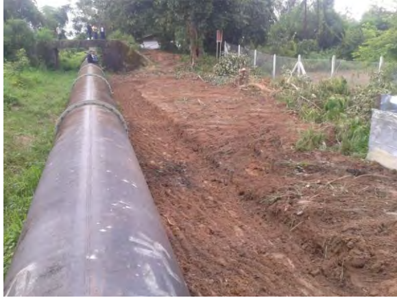
Gyobyu Transmission pipe(MS)
