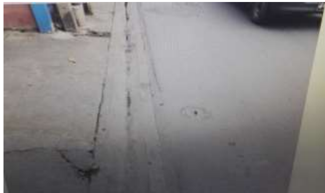
Existance of Gate Valve on the Road
