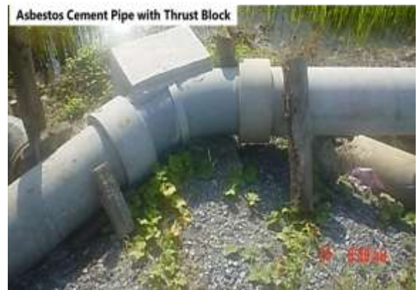
Asbestos Cement Pipe with Thrust Block
