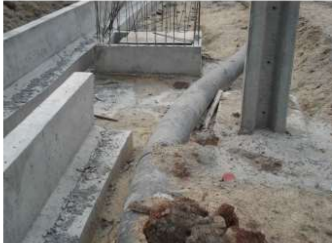
Location causing the pipe laying problem
