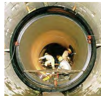
Piping in shield tunnel
