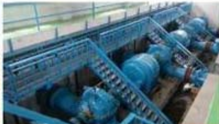
New Pumping Station (2007) at Yegu Pumping Station
