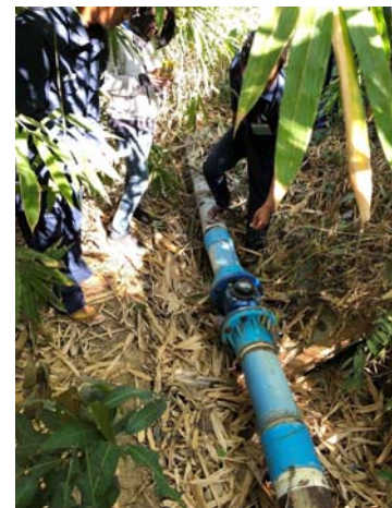
Service connections to Bago T/S
