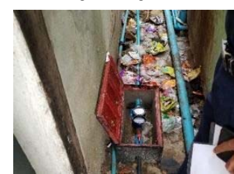
New meter with Meter Box
