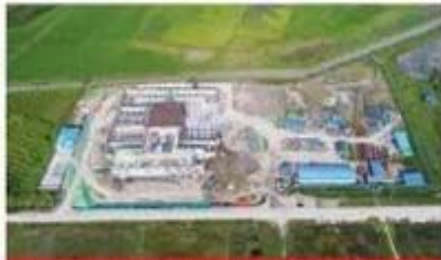
Service Reservoir for Zone (7) in Dagon Myathit (South) Township
