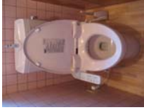
Flush toilet : about 5 Little
