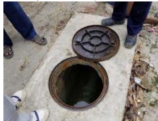
Flow meter Chamber
