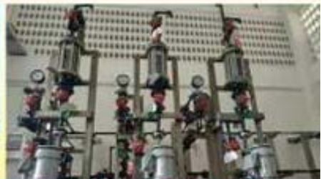
New Chlorine Dosing Facilities
