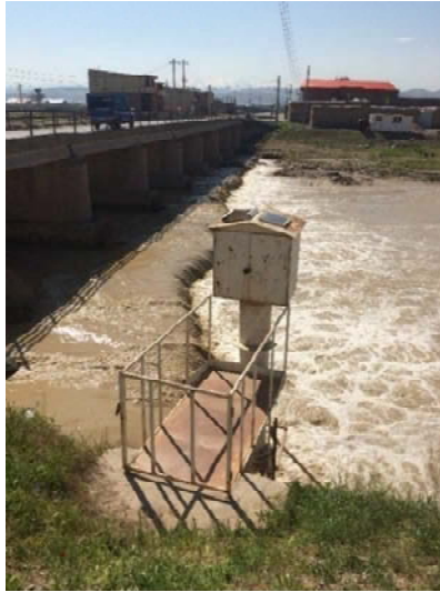
Figure 3.2.17 Akhola Hydrological Station
