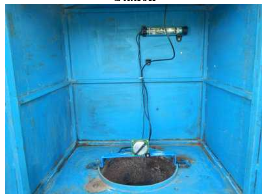
Logger Installed in Sonate Hydrological Station
