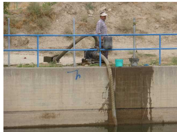
Operation condition of underwater pump for intake
