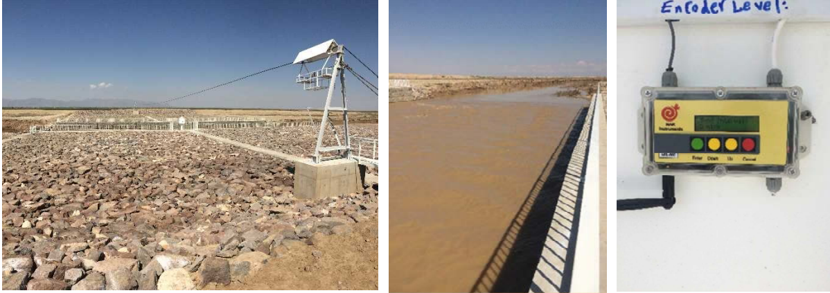
Khor Khor Hydrological Station (No. 11 in Figure 2.4.1)
