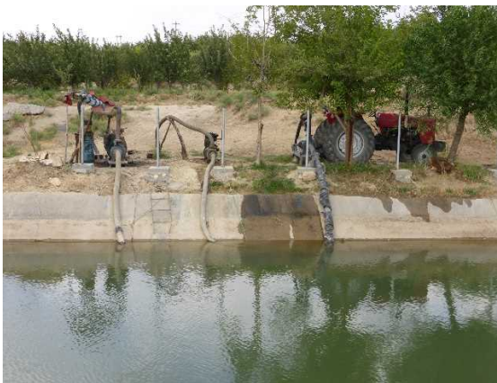
Installation condition of underwater pump for intake
