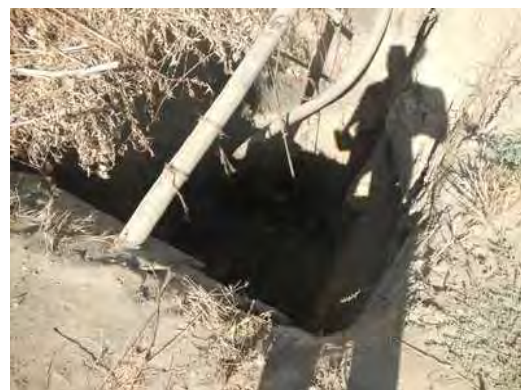
Well installed nearby Simine Rud Hydrological Station
