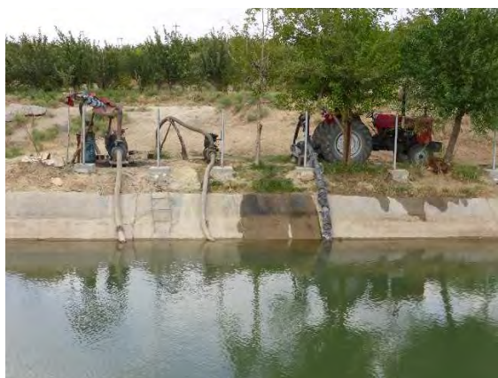
Installation condition of underwater pump for intake
