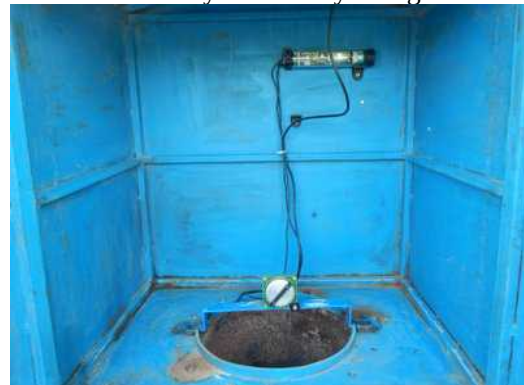
Logger Installed in Sonate Hydrological Station
