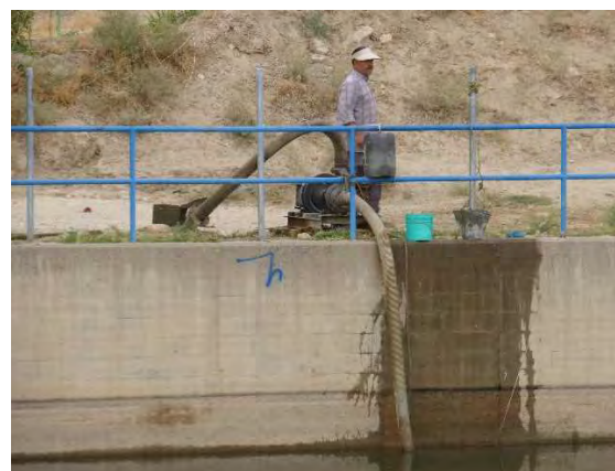
Operation condition of underwater pump for intake
