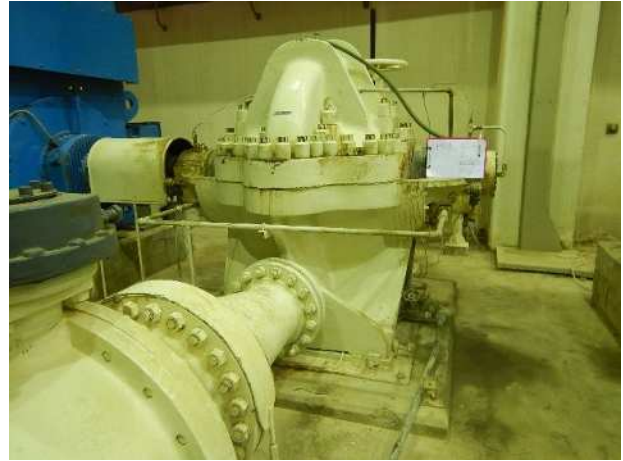
Single-stage centrifugal pump
