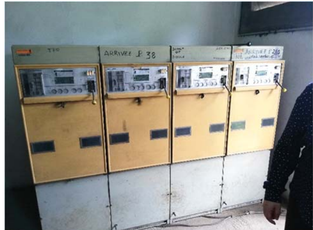
(Switching gear panel)
