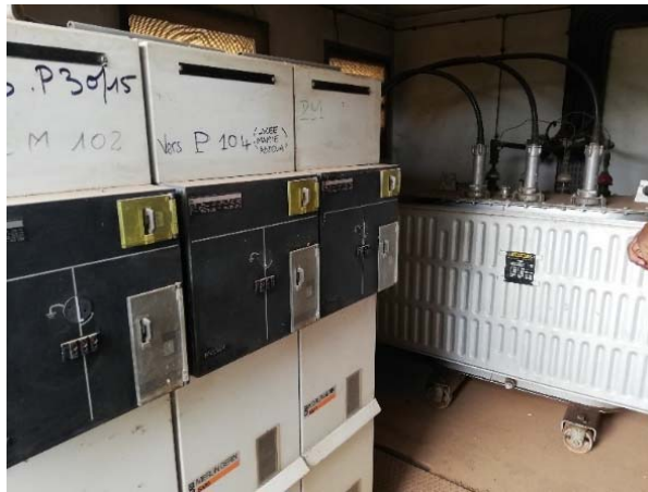
Fig. 4.3-11 An example of insufficient expansion space
