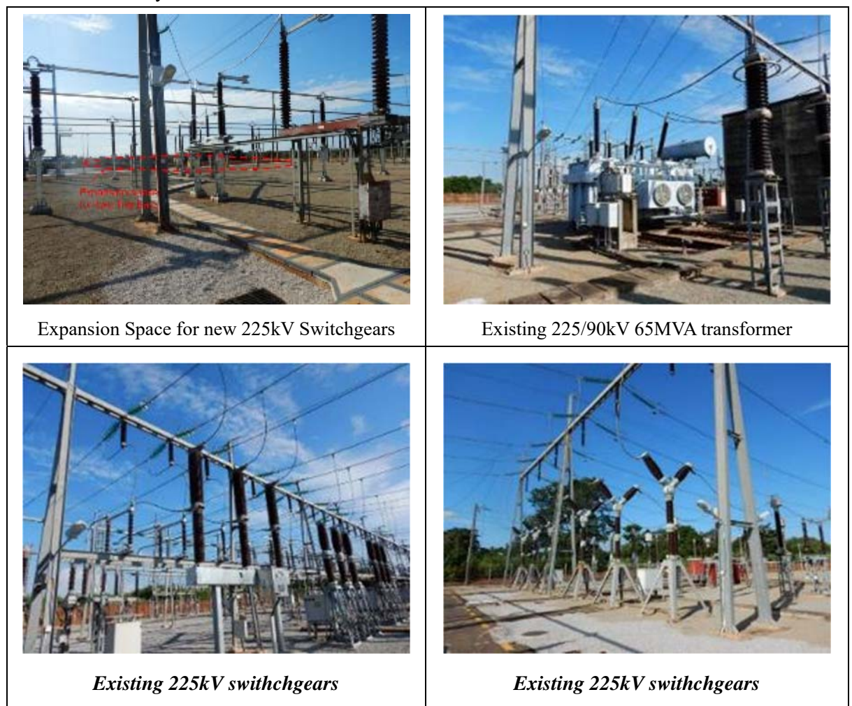
Fig. 4.2-9 Photos of Bouake2 substation
