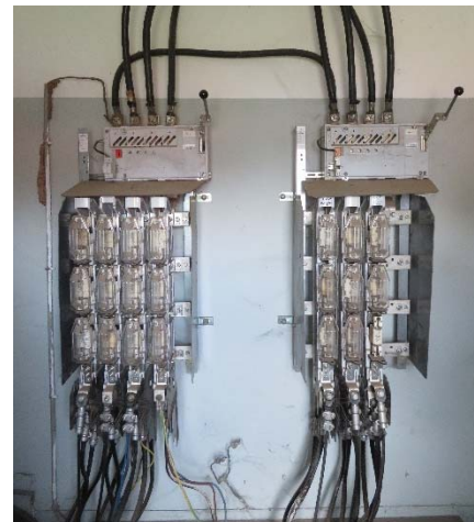
(Low voltage distribution board)
