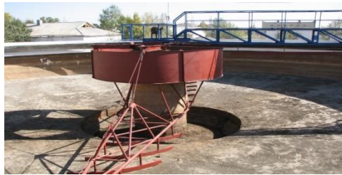
Gravity Sludge Thickener
