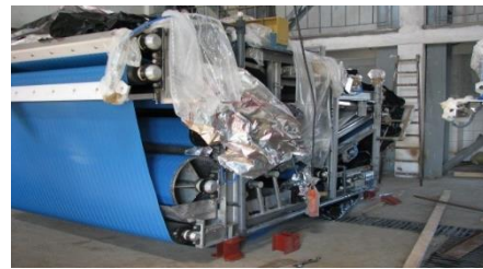
Sludge Dewatering Machine
