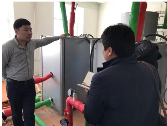
Main body for geothermal heat pump
