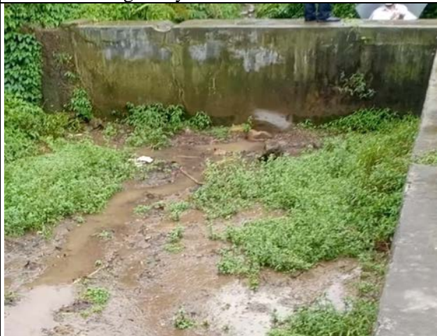
No. 9: Existing Water storage tank but water cannot be stored in this tank due to leakages in many points.
