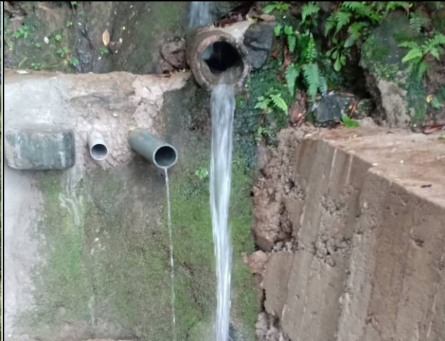
No. 4: Existing water source namely Rawan Ka Ban.
