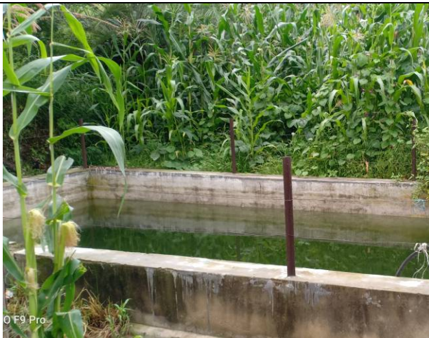
No. 5: Existing water storage tank of an individual farmer from this he is able to irrigate his nearby fields.
