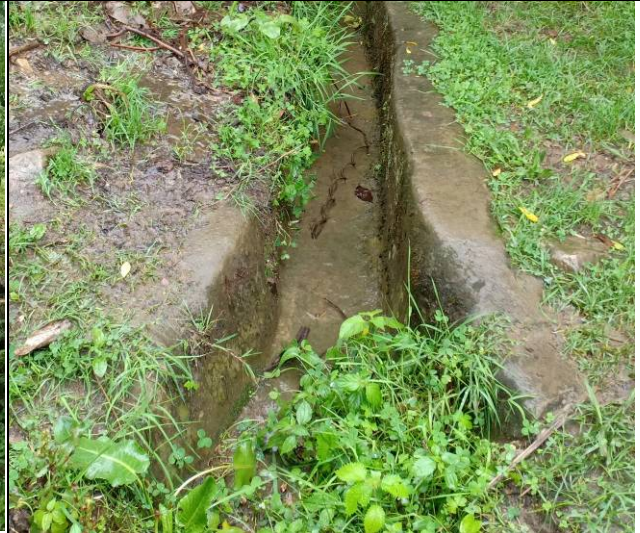
No. 8: Existing channel which is damaged at most of the places.
