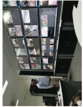
CCTV monitoring panels
