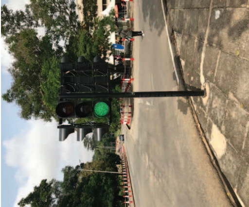
Traffic signal installed at shuttle intersection KNUST
