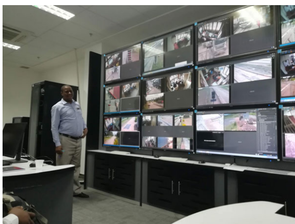
CCTV monitoring panels
