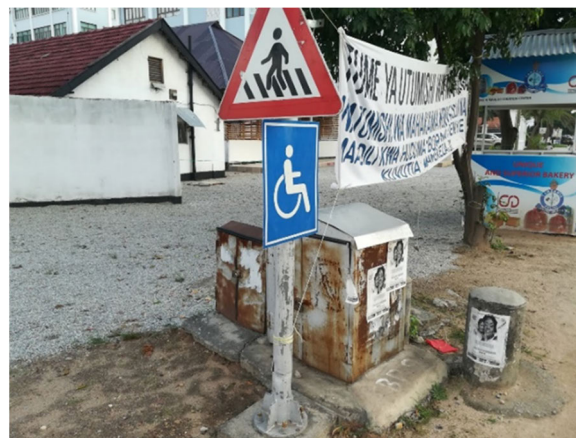
Control box in Ndasha
