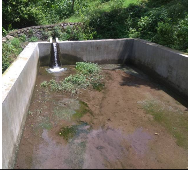
No. 7: Existing water storage tank of approx. 15000 ltrs capacity.
