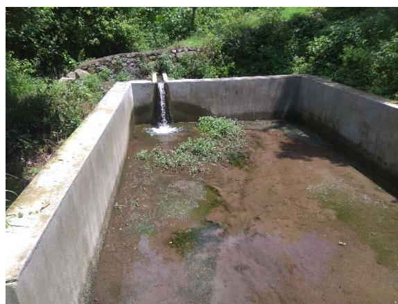
View of the field survey on existing water storage tank at village Chanjota, G.P Panjain Khurd, District Bilaspur
