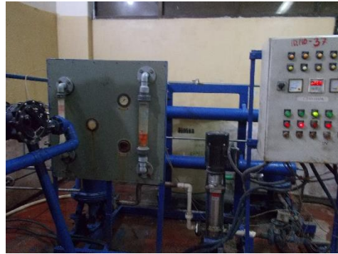
Water treatment with RO (reverse Osmosis)
