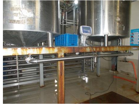
Rusted foot stool
