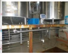
Trestles are corroded
