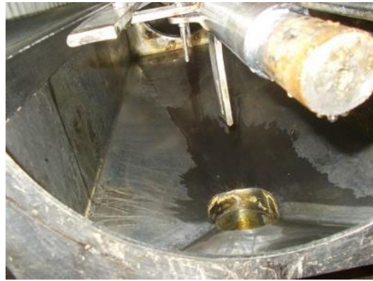
Water residues in a processing machine due to inappropriate maintenance
