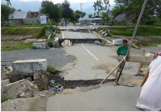
Collapse of Road near Liquefaction Area
