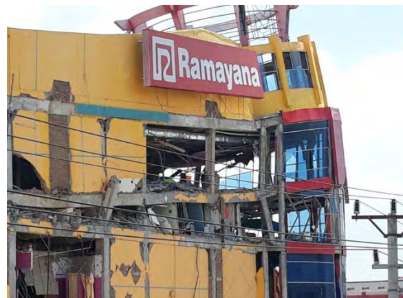
Figure 57 : Inappropriate design of column and material
