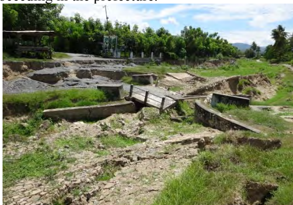
Destroyed irrigation canal in petobo area
