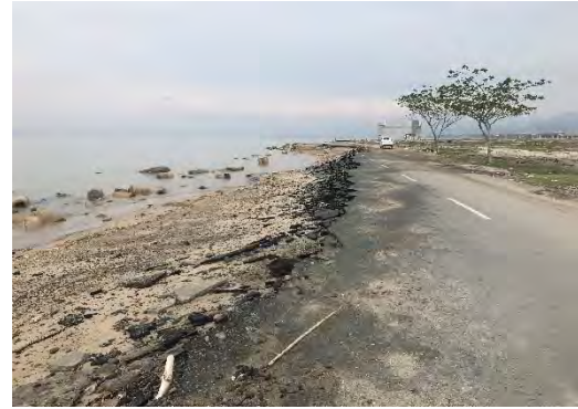
Damaged Road Surface by Tsunami
