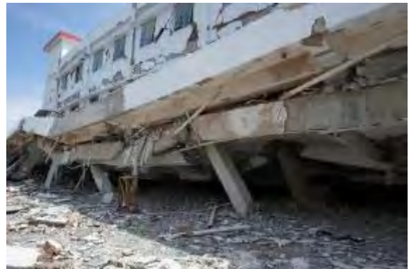
After Earthquake: Totally damage
