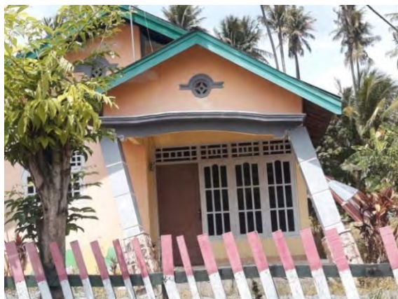
Figure 62 : Tilting column of house
