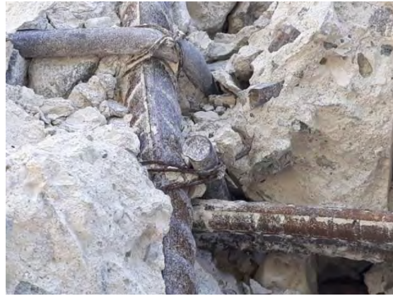
Figure 53 : Inadequate stirrup in Rusunawa Lere
