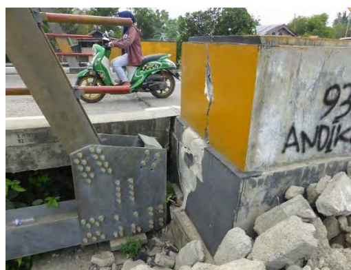
Hit of Girder on Abutment
