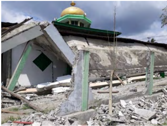
Figure 58 : Collapsed of Mosque
