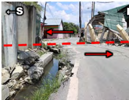
Figure 39 : Surface rupture at 20181102-6 site, Cemara str. Donggala Kodi districts.
