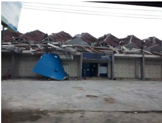
Figure 60 : Damaged Roof of Stores
