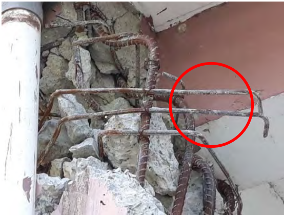
Figure 54 : Inadequate stirrup in Rusunawa Lere
