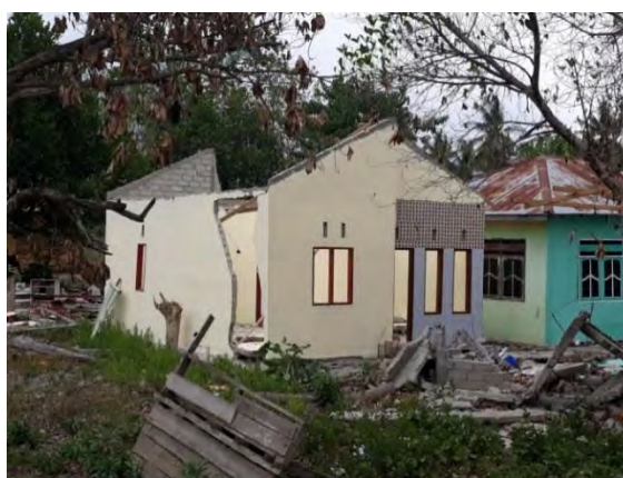
Figure 65 : Partial Collapsed of House
