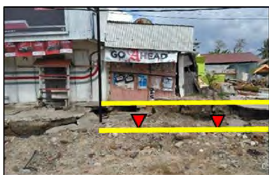
Figure 66 : Collapsed by Land Subsidence
