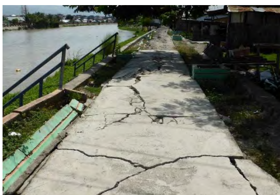
Cracks on Top of Banks
