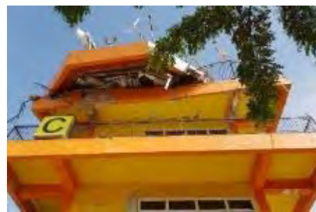
Destroyed control room
