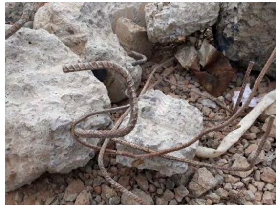
Figure 51 : Too small reinforced bars used in Roa Roa Hotel
