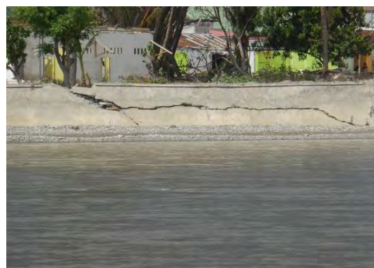
Collapse of Revetment
