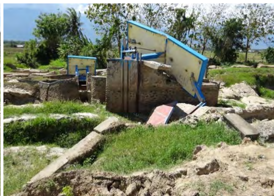
Destroyed diversion work in Jono Oge area
