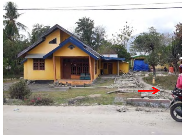
Figure 61 : Tilting column of house and moving fence
