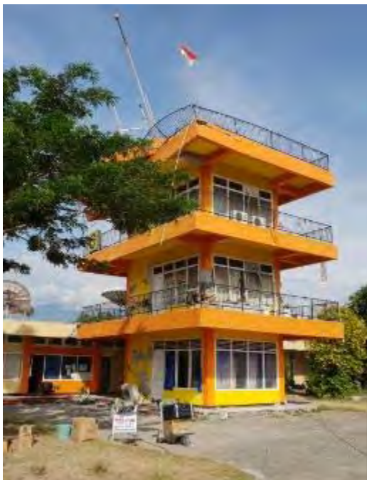
Due to earthquake, the control tower had critical damages
