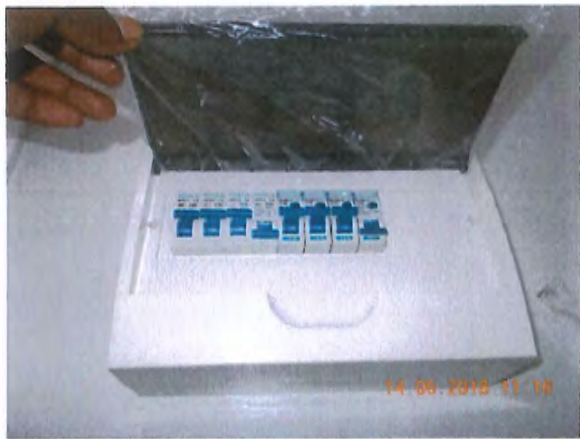
Plate 15. Electrical distribution board
