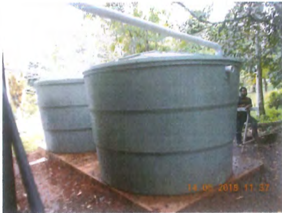
Plate 13. 2 x Rain water 'tuffa' tanks
