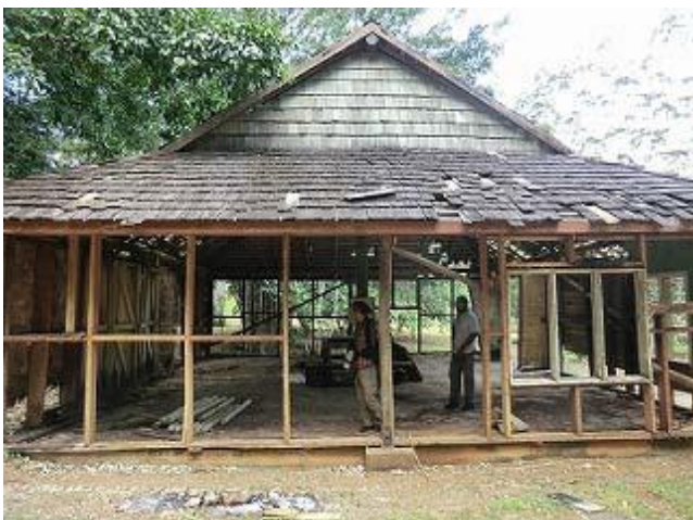
Photo 3: Information center is deteriorated at VNP (VNP).
