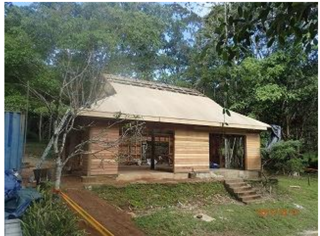
Photo 8: The renovation of the existing information center is ongoing. Photo showing side view (VNP).
