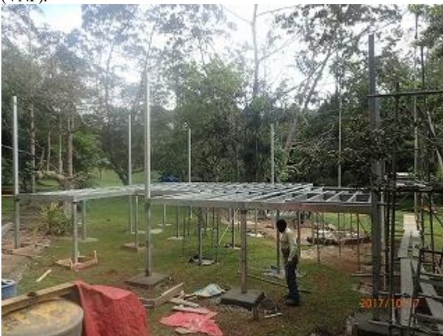
Photo 9: The construction of the new information center with steel posts and beams (VNP).
