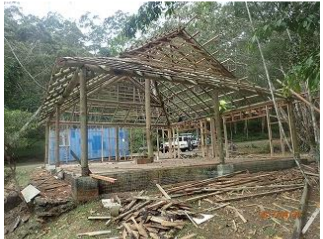
Photo 4: Roof repairing work is progressing for renovation of Old Information Center (VNP).
