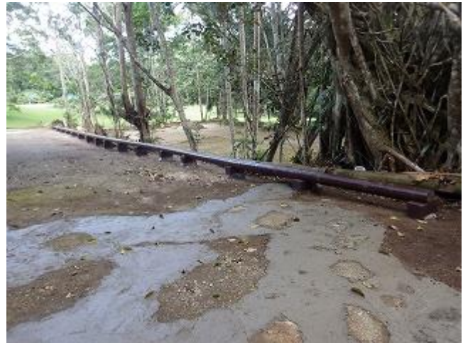
Photo 10: Car stop piles were installed at the parking area in Varirata National Park (VNP).
