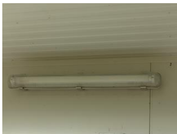
Photo 6: Security light was installed at the front of the Tahira Marine Office (Tahira).
