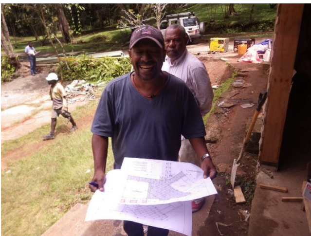
Photo 5: Mr. Howard of CEPA-JICA Project team using the draft floor design of the wooden decking to make measurement at the construction sites (VNP).
