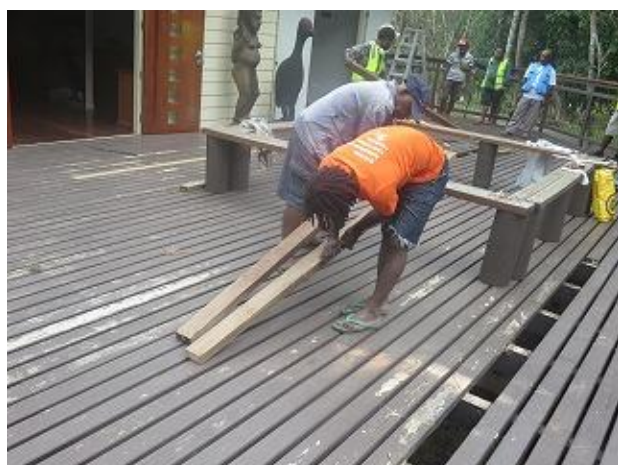
Photo 5: Mr. Tati of park staff, sanding woods to repair wood decking at Varirata National Park (VNP).
