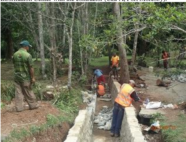
Photo 11: Local construction contractor, repairing the drainage of parking area in Varirata National Park (VNP).
