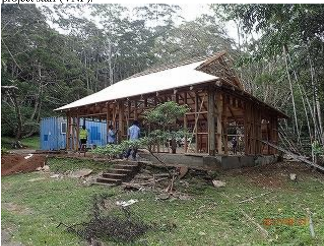
Photo 3: Renovation of old information center is ongoing and once completed will be part of new complex as a auditorium (VNP).
