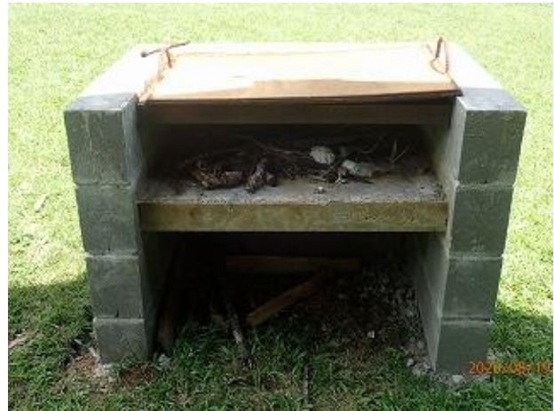
Photo 8: Barbecue stands at main picnic area are renovated by CEPA and UNDP GEF 5 Project (VNP).
