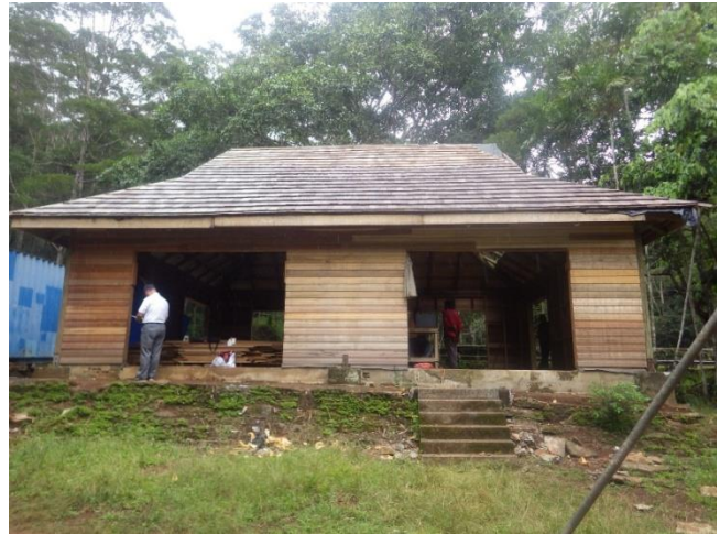
Photo 2: Mr. Sakano of JICA inspecting the renovation work of the old IC (VNP).
