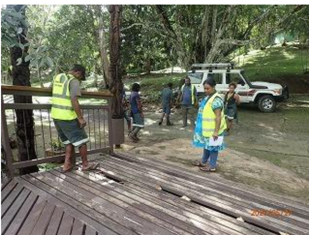
Photo 11: Park rangers and Ms. Saina of JICA, checking the rotting timbers of wood decking at information center complex (VNP).
