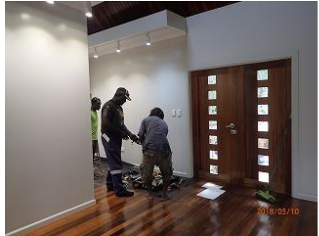
Photo 2: Workers of Rhodes PNG Ltd.(sub-contractor) finalizing interior of New Information Center (VNP).
