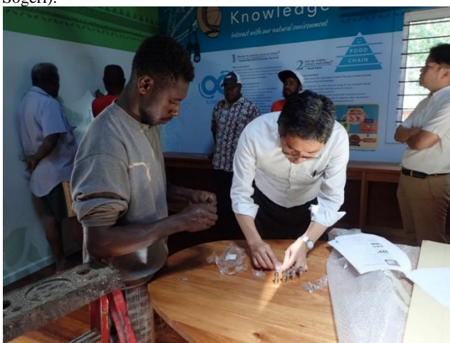
Photo 5: Mr. Hoshiiai of JICA giving instruction to local contractor Color Boys on the installation of picture walls in new IC (VNP, Sogeri).
