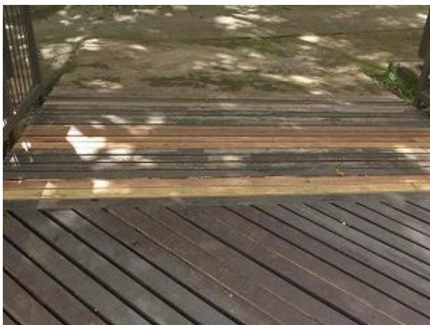
Photo 11: Wood decking at Information Center Complex was repaired by park rangers (VNP).
