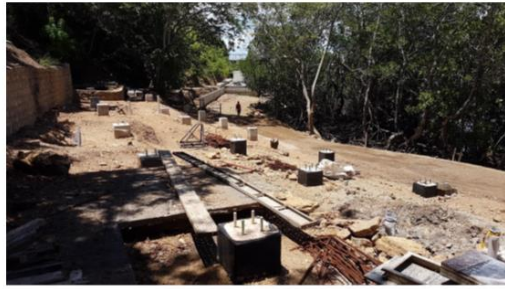
Hill Side Bungalows (HSB) type B number O1 and O2 completed for concrete foundation works
