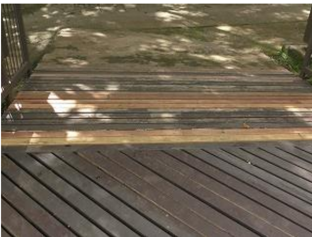
Photo 11: Wood decking at Information Center Complex was repaired by park rangers (VNP).
