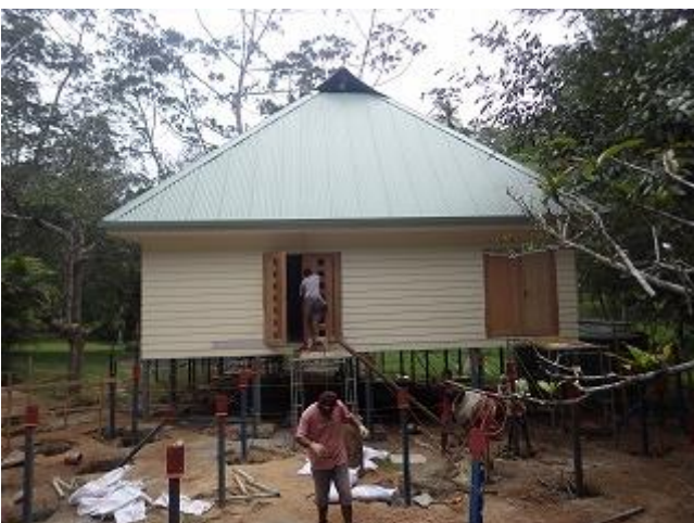
Photo 5: A worker of Rhodes PNG Ltd.(sub-contractor) installing a door for new information center (VNP).
