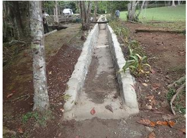
Photo 2: Repairing the drainage in Varirata National Park has successfully been completed (VNP).
