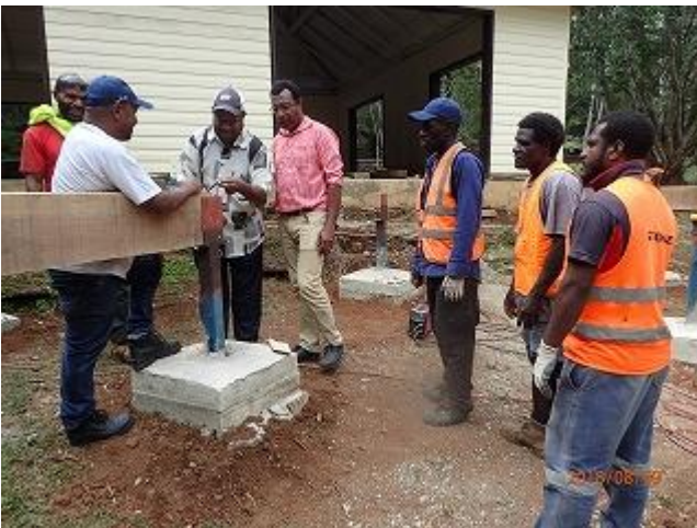
Photo 3: CEPA-JICA project team confirming progress of wood decking for Information Center Complex (VNP).
