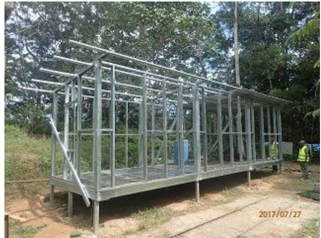
Photo 8: Construction company for new Information Center, constructing base camp kit house in Varirata National Park (VNP).
