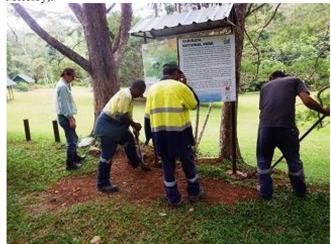
Photo 6: Mr. Imai of JICA, supervising the contractors installing a signboard at the main picnic site of the park (VNP).
