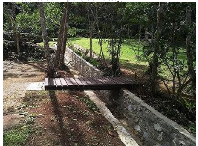
Photo 4: Newly installed trench and wooden foot bridge, ready to be used by visitors (VNP).
