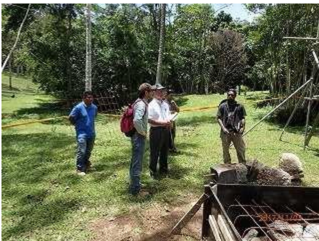
Photo 5: Mr. Sakano and Mr. Imai of JICA inspecting progress at the construction site of new information center (VNP).
