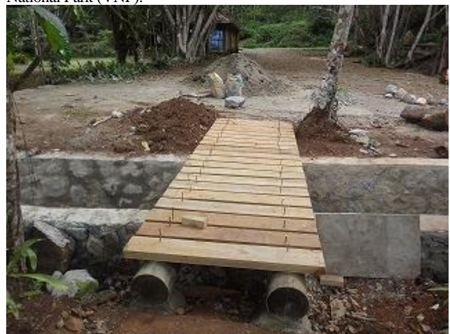
Photo 12: Several wooden foot-bridges in Varirata National Park is in the middle of construction (VNP).
