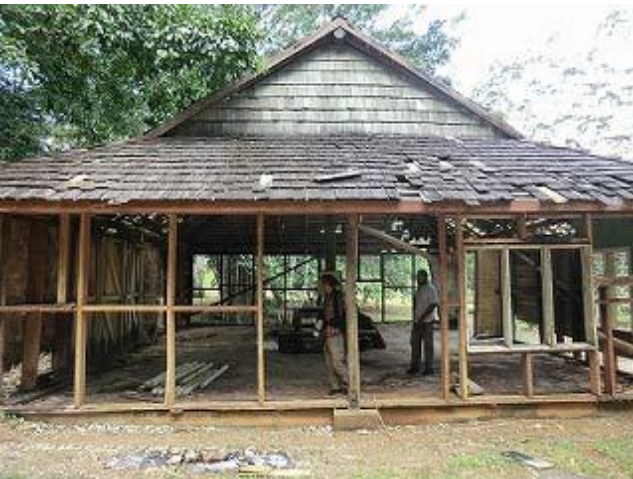
Photo 3: Information center is deteriorated at VNP (VNP).
