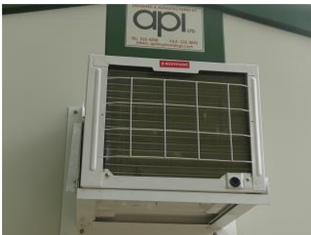
Photo 5: The Air condition unit was installed at Tahira Marine Office (Tahira).
