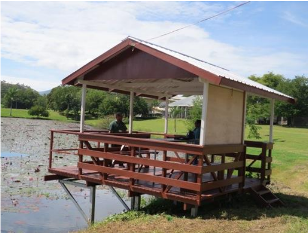
Photo 1: Extension work of the bird watching shelter at Pacific Adventist University was completed (PAU).
