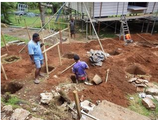
Photo 11: Local contractor digging holes for installing support piles of wood deck (VNP).
