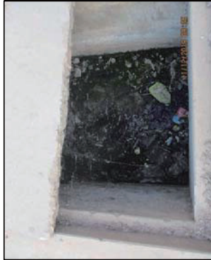
Manhole Sludge and garbage
