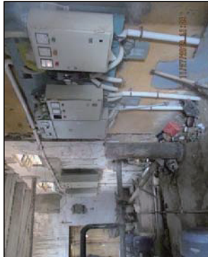
Motor Control panels
