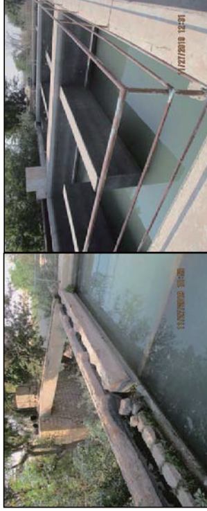
Intake Channel to mixing tank
