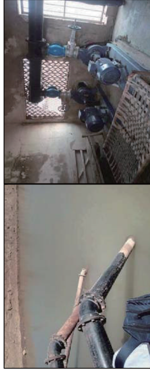
Pump's Suction from Canal
