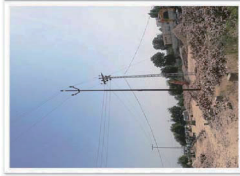
11kV Overhead Feeder
