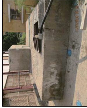
Water Tank No. 2 for Hospital Building
