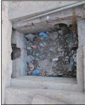
Manhole filled with garbage & dust
