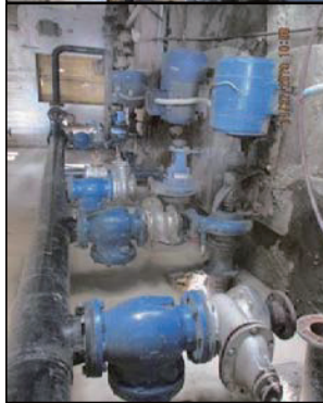
Currently Installed pumps
