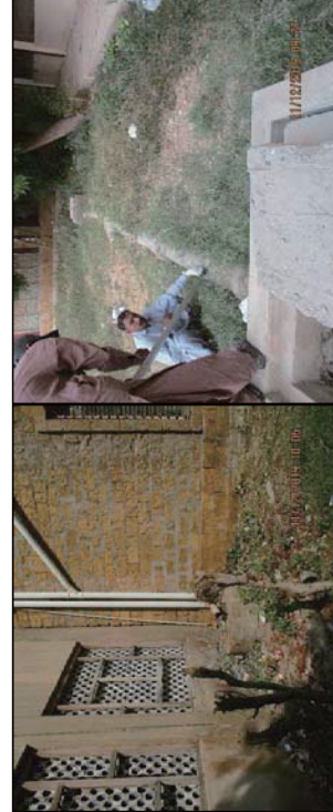
Building pipe connection to manhole
