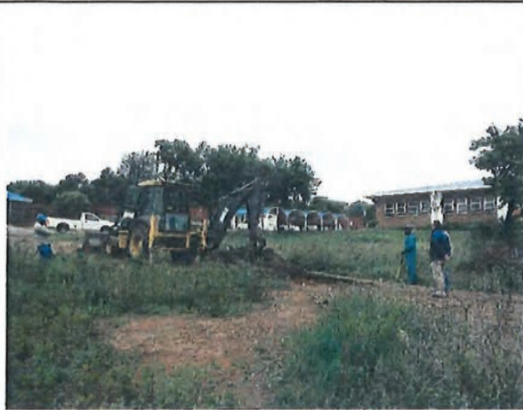
Photo-1 Confirmation of Underground Pipe at Candidate Location of Training Yard in IBTC
