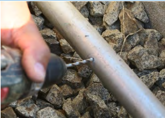
Photo-101 Yard Construction (Leak Hole on Steel Pipe)
