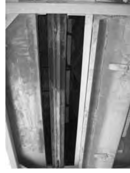
Working Water Shower System
