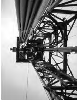
Top Drive System installed Mast
