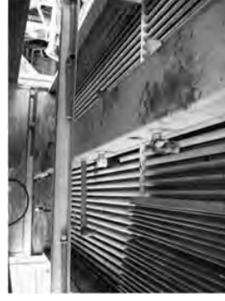
Water Shower System (In side View)
