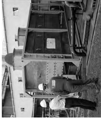
Mud Cooling Tower (Outside View)
