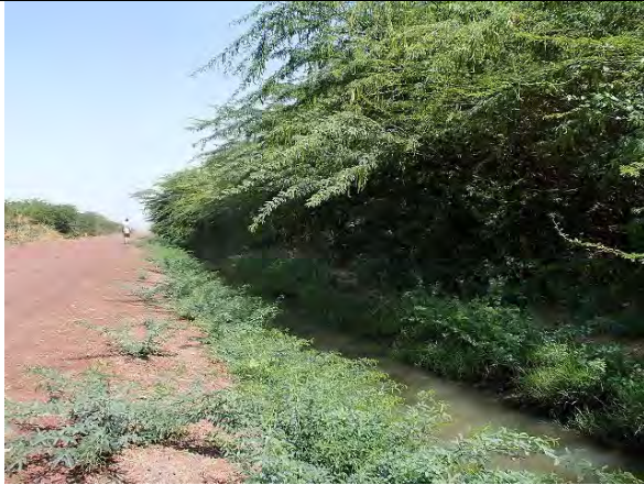
9. .SC1-5. Deep Bushes on the right bank of the canal, and the canal is close to farm land, so it seems to be difficult to construct pipeline on right bank.
