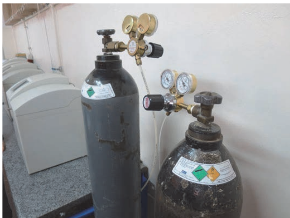
Photo 2.3-33 Installation Condition of Nitrogen Gas
