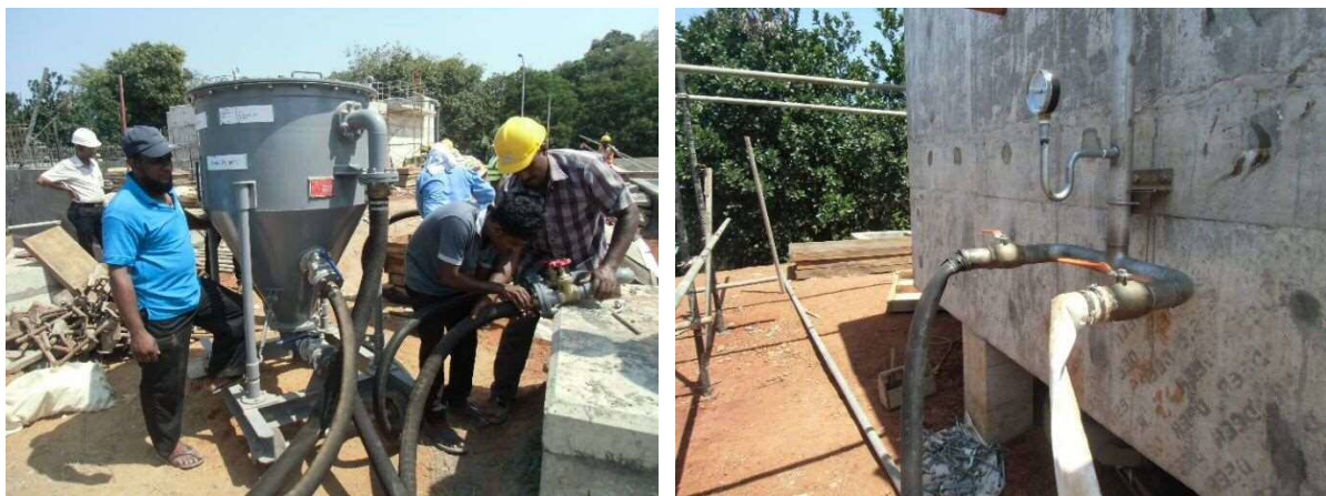
Figure 2-13 Setup of Sand Separator Tank (Left) and Connection Point of Pressure Water (Right)
