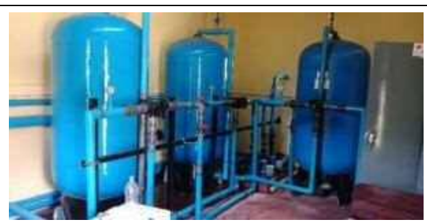
Photo 5-3 Sewage filtration facility
