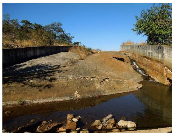
Damaged Spillway of Sasa Dam
