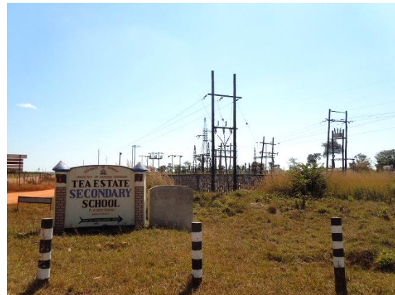
An electric substation along the Trunk Road in the northern part of Luena FB.
