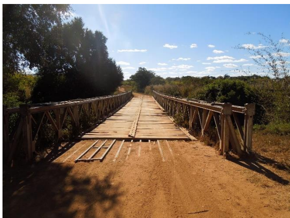
Damaged Luombwa Bridge crossing Luombwa River
