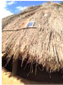
Solar panel on the roof of the meeting place in the FB. Farmers use electricity to charge their mobile phones.
