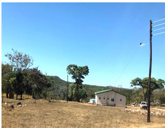
Hydropower station and power lines outside the FB (1MW)
