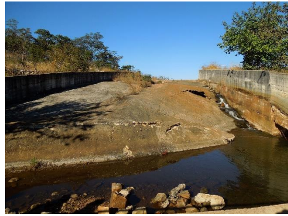
Damaged Spillway of Sasa Dam
