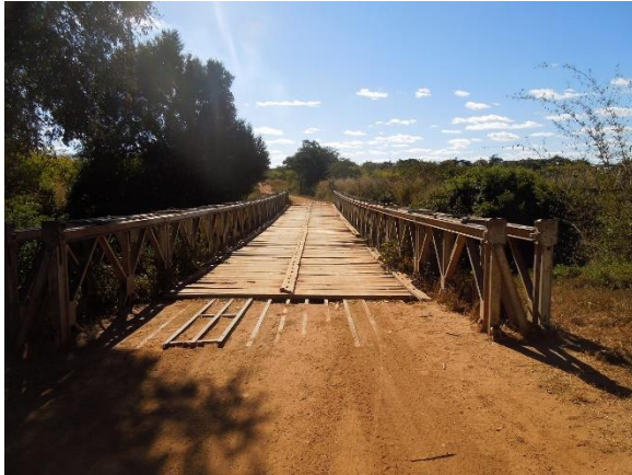
Damaged Luombwa Bridge crossing Luombwa River
