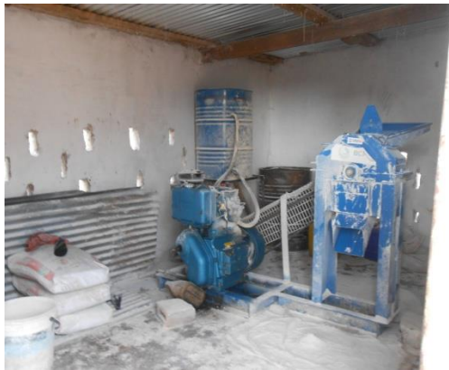
Maize milling machine driven by a diesel generator
