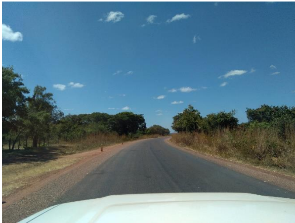
Road surface conditions of the two-lane trunk road north of Luena FB (from Kawambwa town to Muporokoso)
