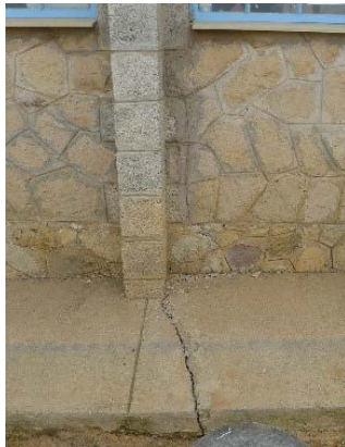
Defect status: Cracks at concrete slab of south outer side of building
