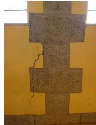
Defect status: Cracks at Teachers room internal wall
