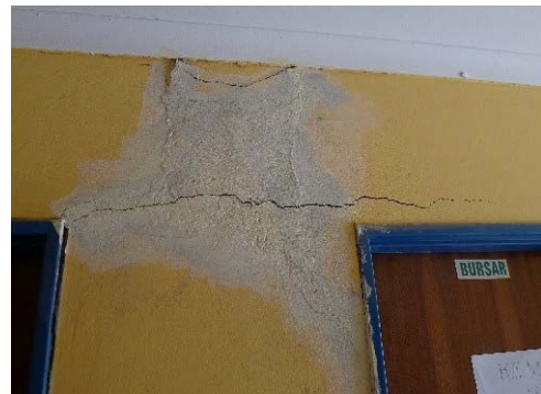
Defect status: Repaired by the School crack occur again after repair
