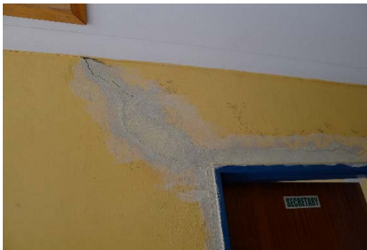
Defect status: Repaired by the School No crack after repair
