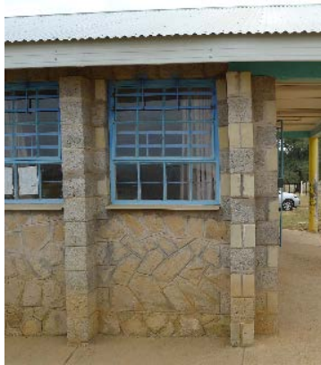
Defect status: Tilted columns
