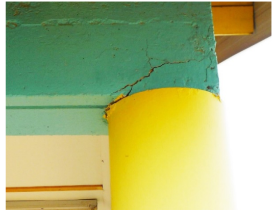
Defect status: Cracks at top of porch column
