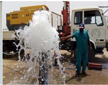
Washing well by air compressor. This work is continued for about 24 hours until the water becomes clean
