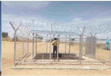
Solar power facility
