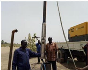
After clean-up of borehole, SWC staff are exchanging old pump to new one.
