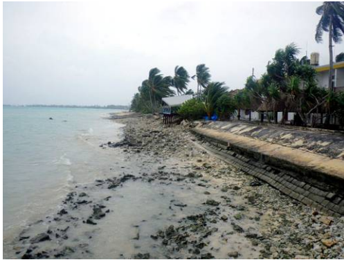
Figure 1.3.1 Damaged Revetment in front of Vaiaku Lagi Hotel
