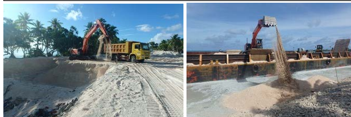
▲ Collection of Sand from Borrow Pit ▲ Placement of sand at Project Site
