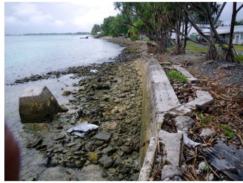
Figure 1.3.2 Damaged Revetment at the North Side of Vaiaku Pier
