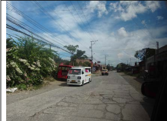
Area B: Barangay Tigatto (no road side drain)
