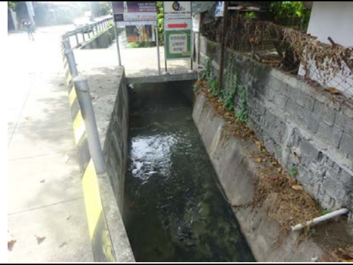
Brgy 20-B: Open drain with discharge from STP
