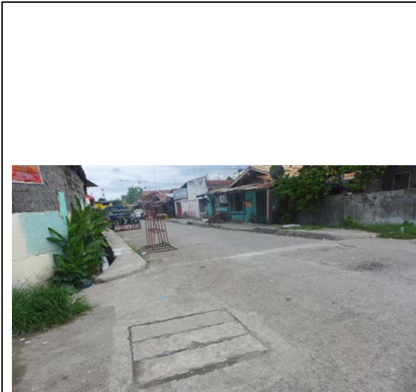
Agdao Dist. Brgy. Vicente Duterte: street, open drain, covered drain, drain manhole
