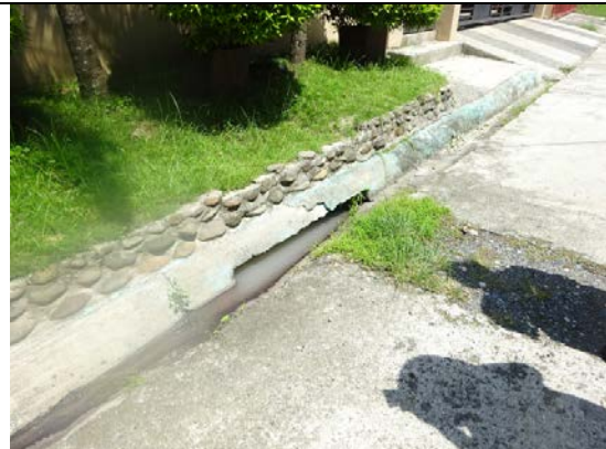
Brgy Buhangin: overflow of gray water from drain due to clogging
