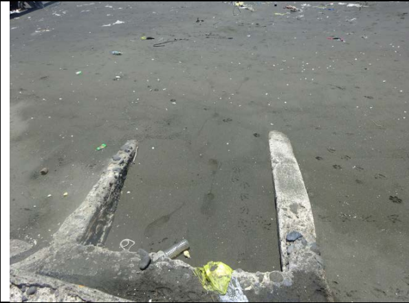
Brgy 76A: clogged outlet of Bucana Main Drain
