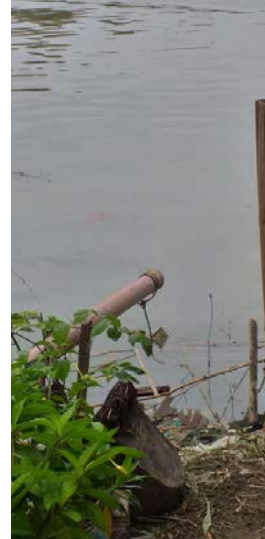
Brgy 2-A: direct discharge of gray water to Davao River
