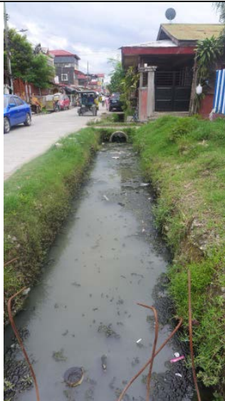
Agdao Dist. Brgy. San Antonio: open stagnant drain
