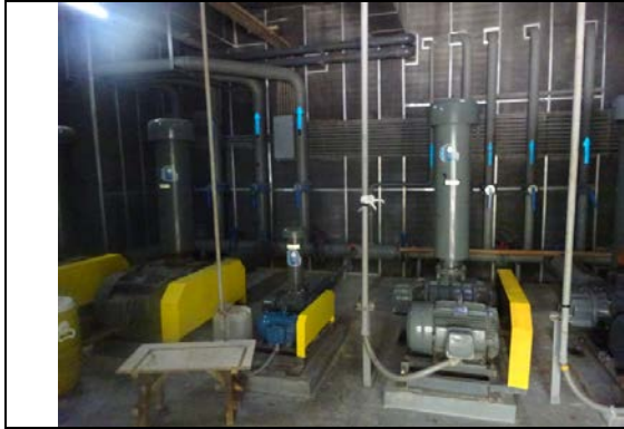
Brgy 20-B: inlet pumping station and blower room in STP
