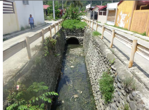
Brgy Tigatto open channel
