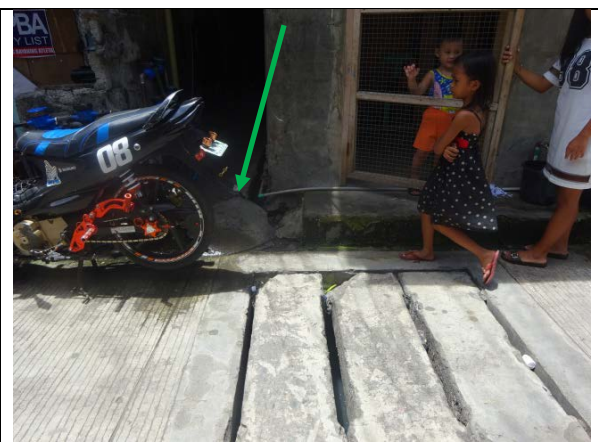
Photo 5.3.3 One Exit of Wastewater from a Congested area in Barangay Tomas Monte Verde
