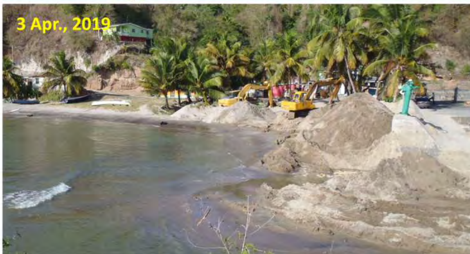
Photo 2-88 Comparison of beach near the sand groin
