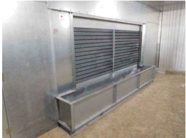
Photo 2-20 Cooling unit for air blast
