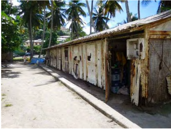
Photo 2-51 Fishing gear lockers (severely deteriorated)
