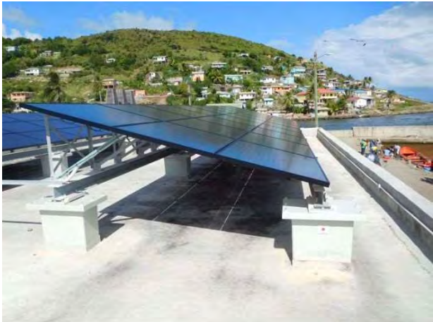
Photo 2-12 Photovoltaic panel and mount
