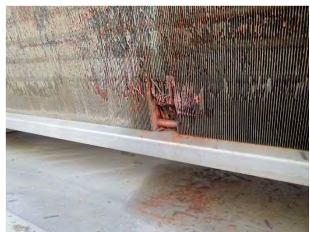
Photo 2-30 Broken part of condenser
