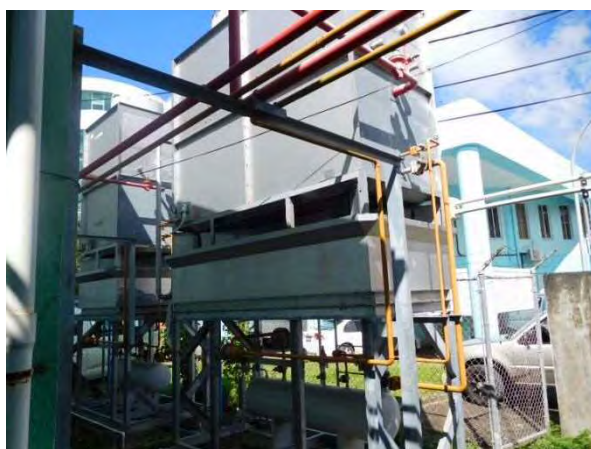
Photo 2-5 Condenser for cold storage and freezing storage
