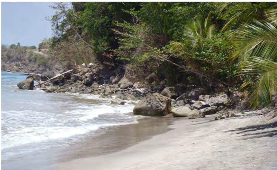
Photo 2-87 Exposed rocks by erosion in the north beach of Choiseul fishing port (April 5, 2019)
