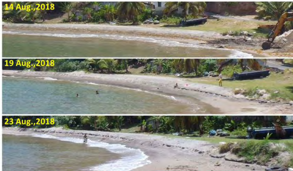
Photo 2-79 Scarp formed by sand being carried to the excavation site
