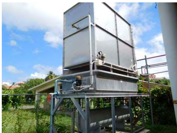
Photo 2-23 Condenser for cold storage and air blast
