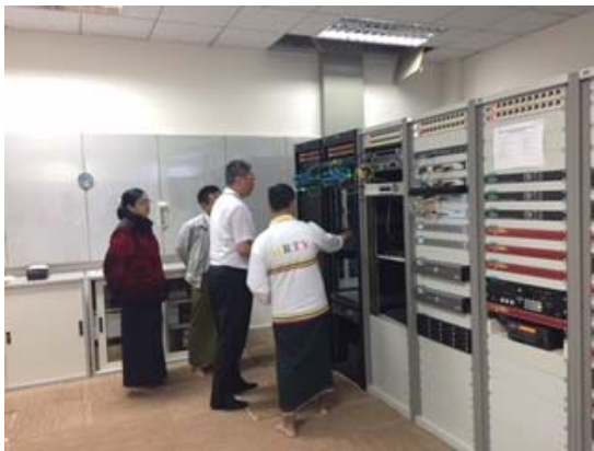
Radio Equipment Checking
