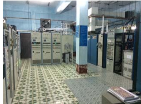
MRTV Taunggyi Transmitting Station (Private TV transmitters are also installed)
