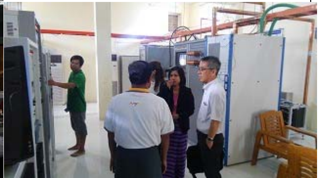
Thabeikkyin Transmitting Station
