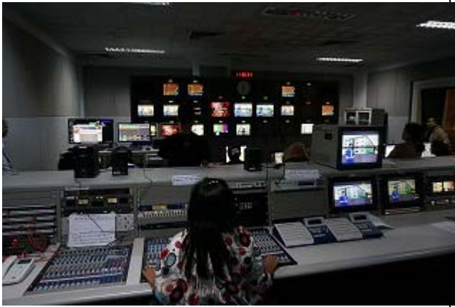
MRTV Sub-Control Room
