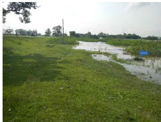
Fig.10 Drainage inhibition by road embankment②
