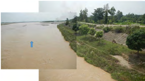
Fig.16 Revetment installed on right bank Revetment is constructed on the dike slope. River water turbidity is high.
