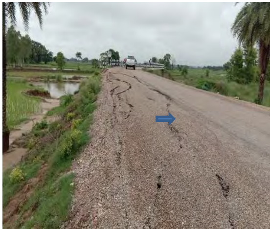
Fig.6 Damaged section of Bagamati – Aruwa Road, Rautahat ①
