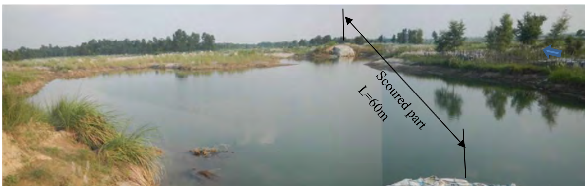
Fig.11 Left bank embankment under repair This part of the levee was scoured with flood overflow on July 2019. This is under repair with sand bags and fabric nets.
