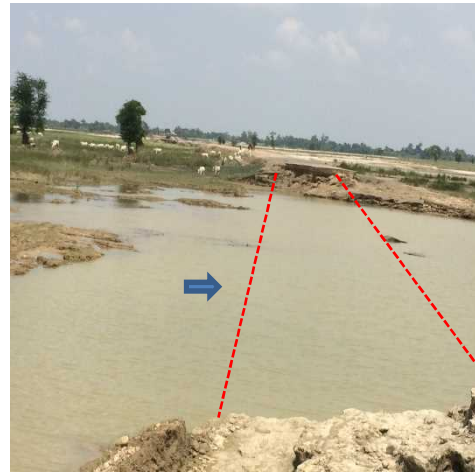
Fig.5 Damaged section of Janakpur – Kaptol Kamal Road, Province 2 ②
