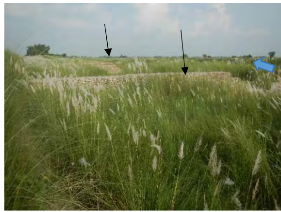
Fig.8 Spur dikes made of gabions② Two spur dikes made of gabions has installed downstream of the scoured part.
