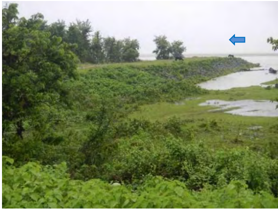
Fig.22 Spur dikes installed on the riverbank① Spur dikes have been continuously installed along the levees.
