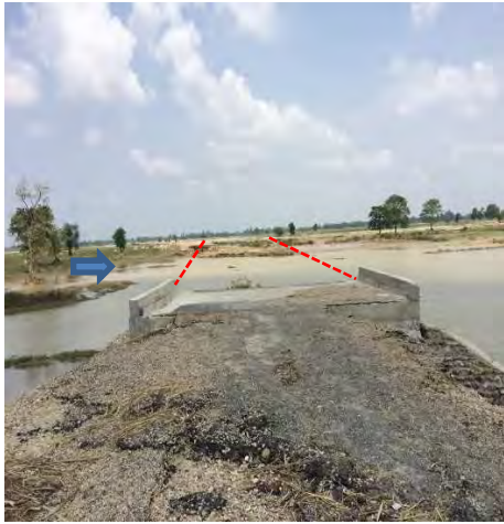
Fig.4 Damaged section of Janakpur – Kaptol Kamal Road, Province 2 ①
