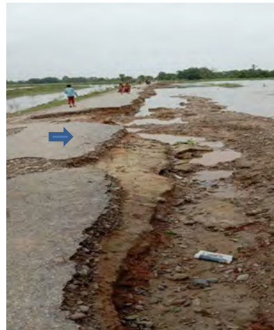
Fig.3 Damaged section of Bagmati – Aruwa Road, Rautahat
