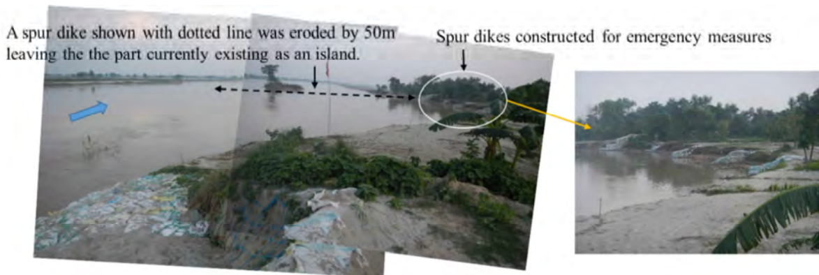
Fig.15 Spur dike scoured by July 2019 flood
