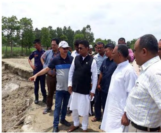
Fig.7 Damaged section of Bagamati – Aruwa Road, Rautahat ②
