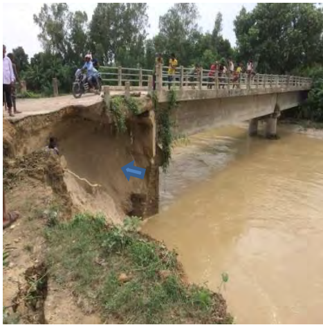
Fig.2 Damaged section of Janakpur – Yadukuha Road, Province 2
