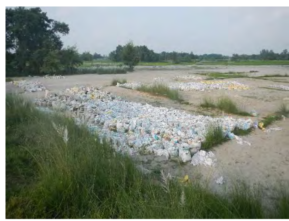
Fig.10 Sand bags in preparation Sandbags have been prepared for repair of scoured part of levee (Fig.12).
