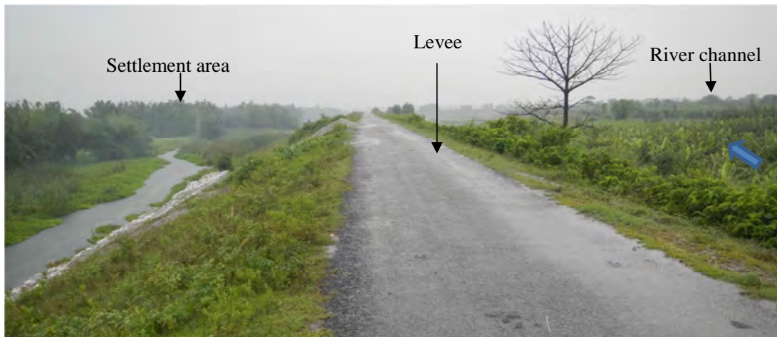
Fig.24 Settlement area lower than river chaneel
