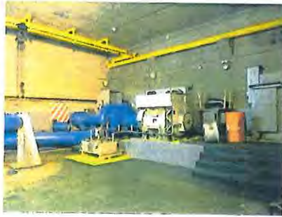
Fig. 2.2.4.3-1 Existing generating facility
