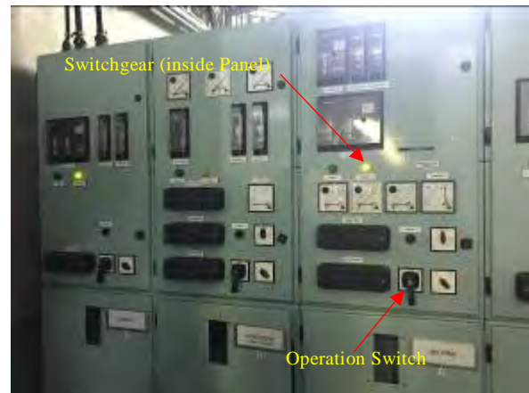
Figure 5-4.7 Existing Katse switchgear
