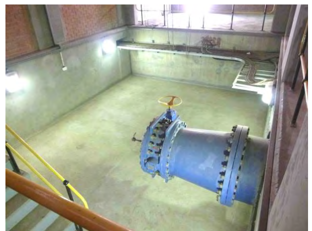
Power generation facility compartment in the Mohale dam discharge valve room
