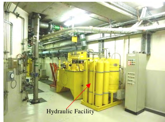
Figure 5-4.23 Turbine pressure-oil equipment
