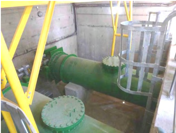
Metolong dam discharge valve room
