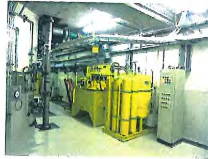
Fig. 2.2.3.4-2 Turbine pressure-oil equipment
