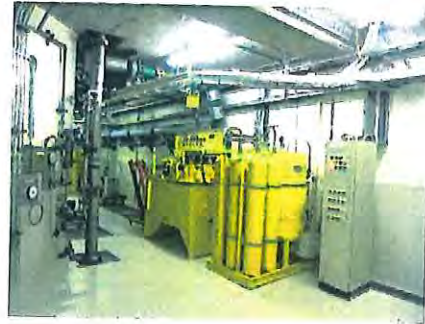
Fig. 2.2.3.4-2 Turbine pressure-oil equipment
