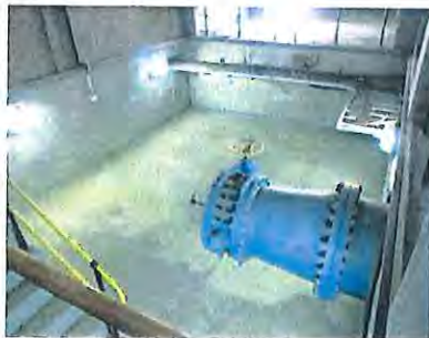
Fig 2.2.2.3-1 Compartment for generating equipment
