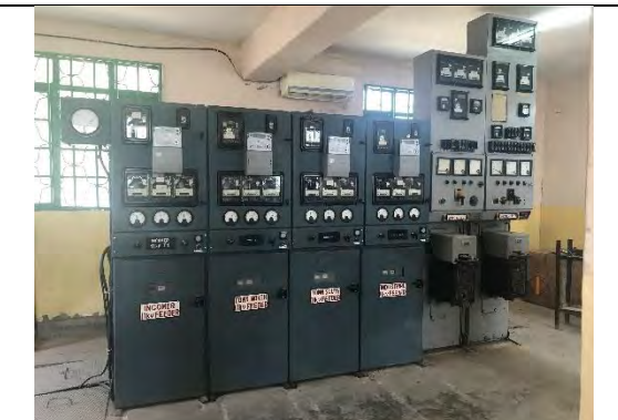
33/11kV Dodoma Town Substation (Control Room)
