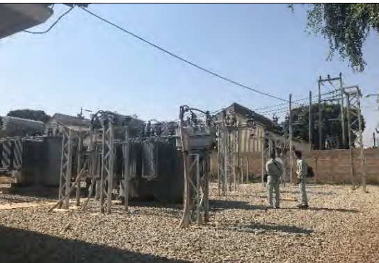
33/11kV Dodoma Town Substation (Switchgear)
