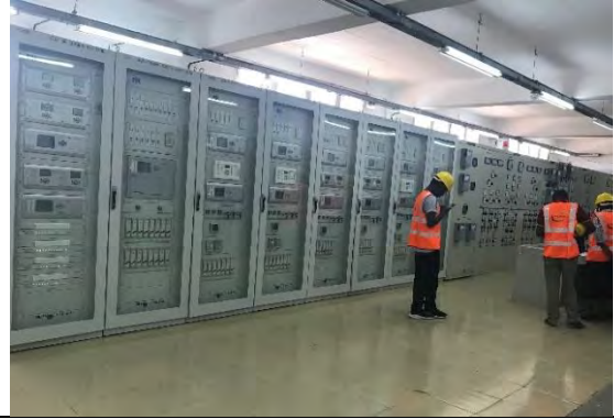
220/33kV Zuzu Substation (Control Room)
