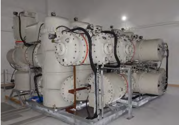
(a) 145 kV GIS for City Center Substation in Dar es Salaam
