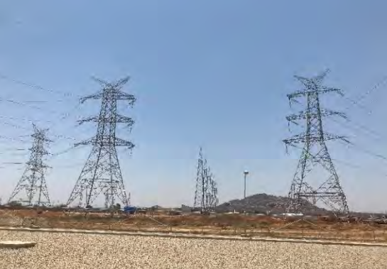
Transmission Lines around 220/33kV Zuzu Substation
