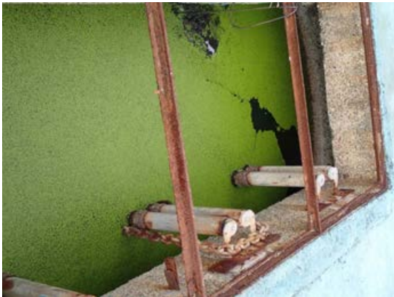
Effluent discharge pumps (Effluent of WWTP is pumped to ocean outfall point of 1.2km offshore.)
