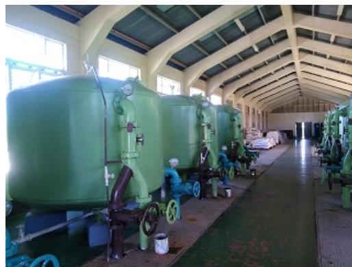
Condition of filters
