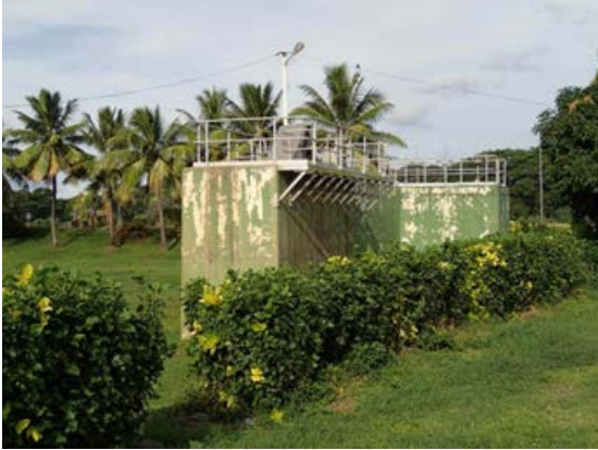
Inflow surge tank (Inflow wastewater is pumped from pumping station in the town center.)
