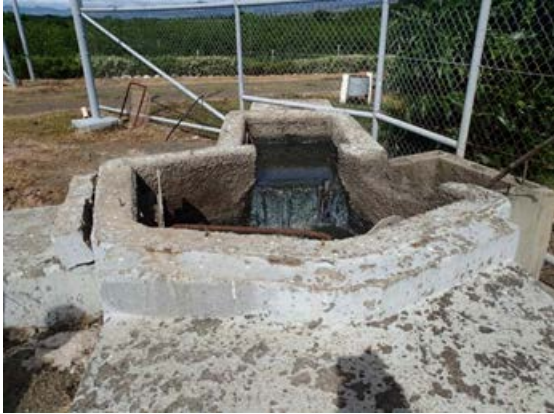
Inlet (Wastewater is pumped from the center of the town. Septic tank sludge is dumped into the inlet.)
