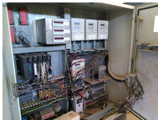
WTP SCADA system not operational
