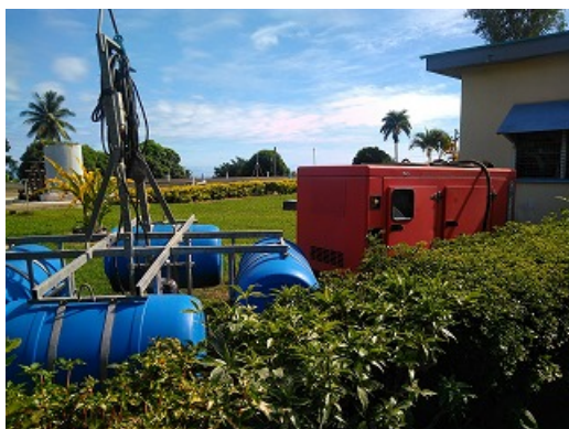
Intake pump of mobile station
