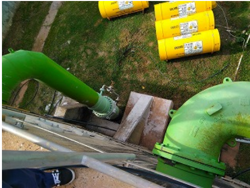
Renewal of inlet regulator (2018)
