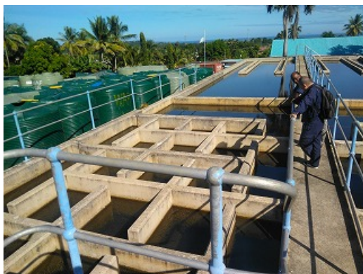
Condition of flocculation tank and sedimentation basin
