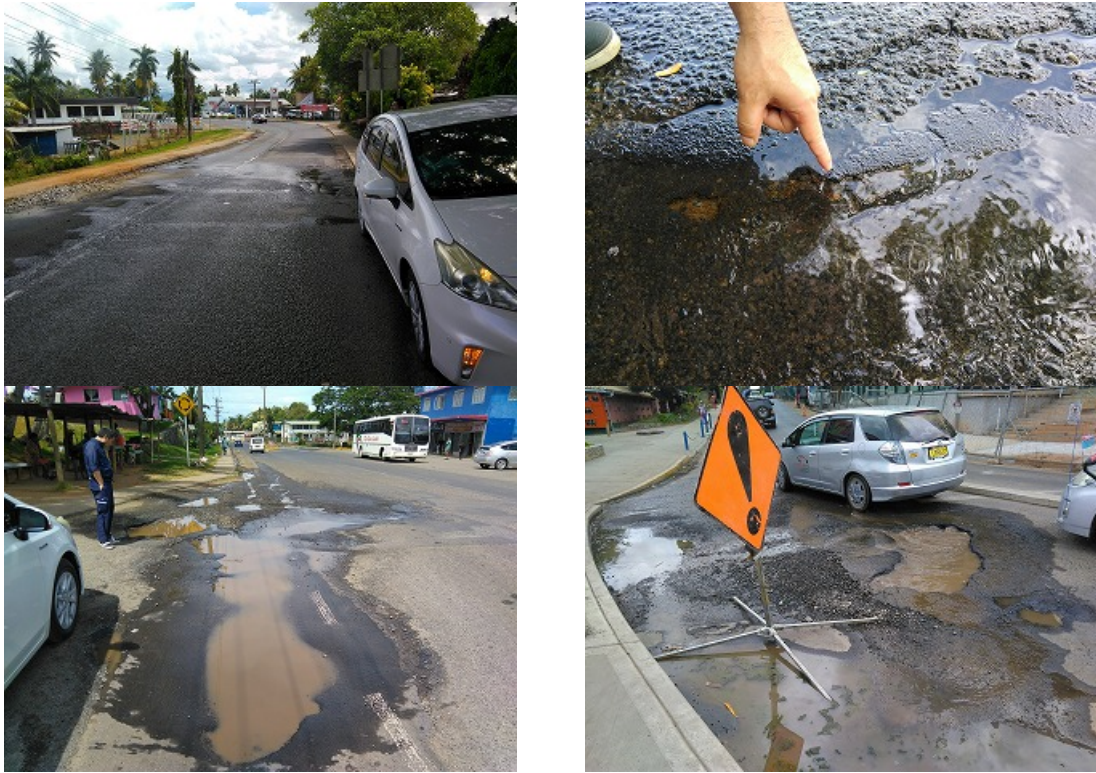
Figure 3-3.21 Leakage Conditions Verified in Nadi Town
