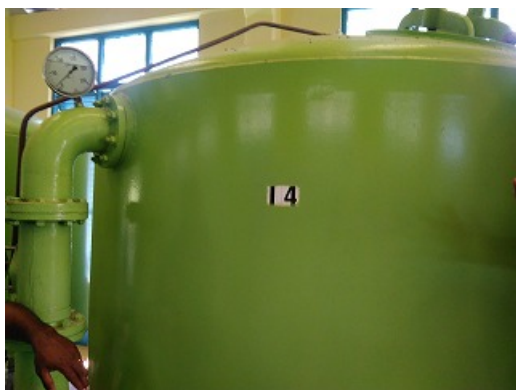
Pressure filter No. 14 malfunctioning
