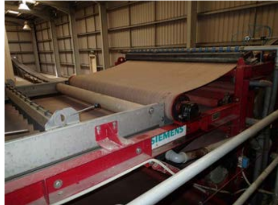
Belt-press dehydrator (Stopped operation due to SCADA trouble)
