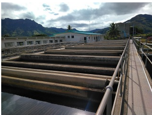
Condition of filter
