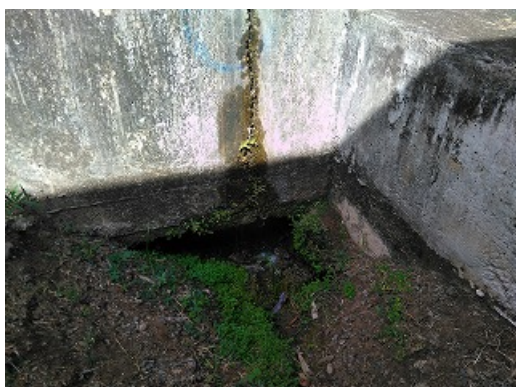
Leakage from crack on floor of distribution reservoir
