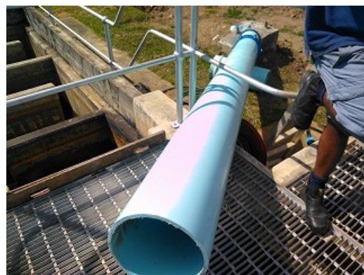
Pressurized main from Nalau Intake (2019)
