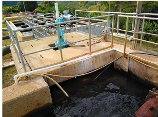
Renewal of inlet regulator (2019)
