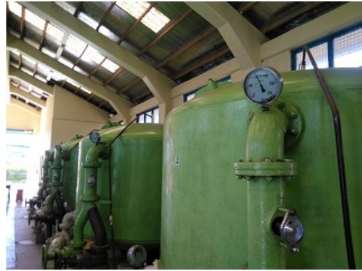
Condition of pressure filters
