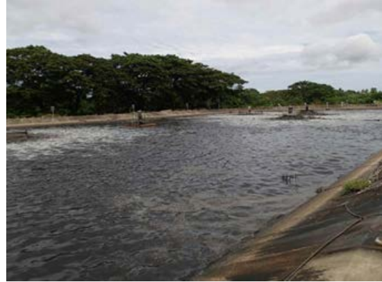
IDEA reaction tank (Floating aerators are set on the tank.)
