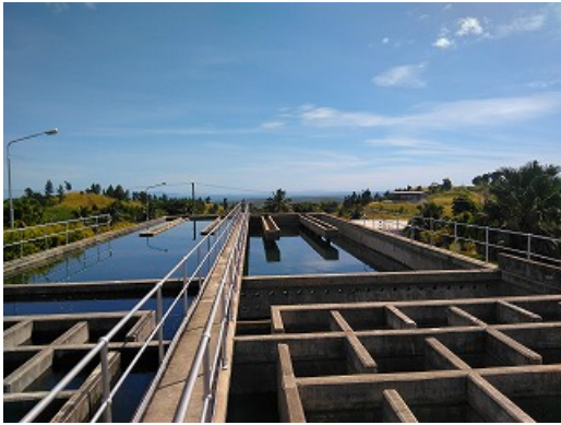
Condition of flocculation tank and sedimentation basin
