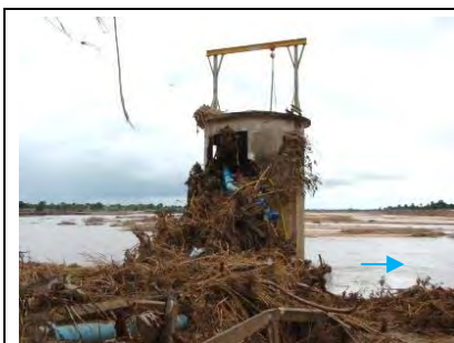
Intake facility for water supply on right bank of Lugela River was damaged
