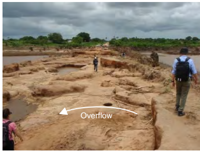
Approach road to Br-1: Crown of embankment was eroded due to overflow
