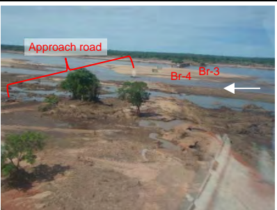
Approach road to Br-4 completely disappeared
