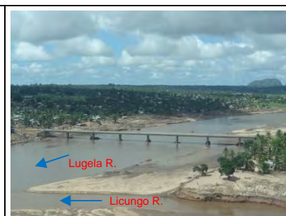
Lugela R. Br: Some railings were washed away due to overflow but traffic is secured after cleaning the debris on the bridge
