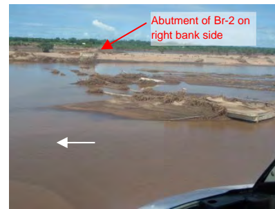
Br-2: Dropped bridge beam
