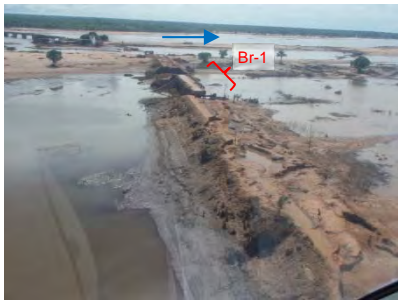
Approach road to Br-1: Crown of embankment was eroded due to overflow
