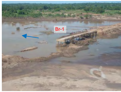
Br-1: Main body is remained but approach roads of the both side were washed away
